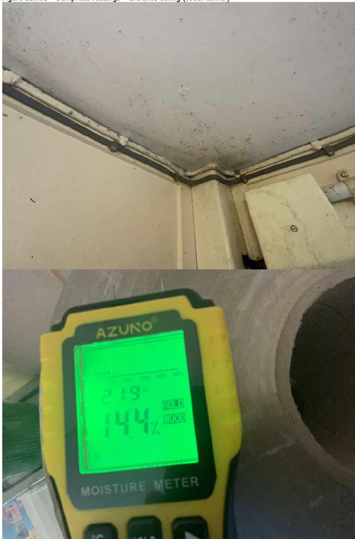
Figure 116.01 – Dampness readings – entrance ceiling (south corner)
