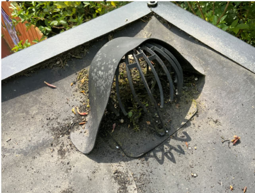
Figure 106 – Blocked roof drainage outlets
