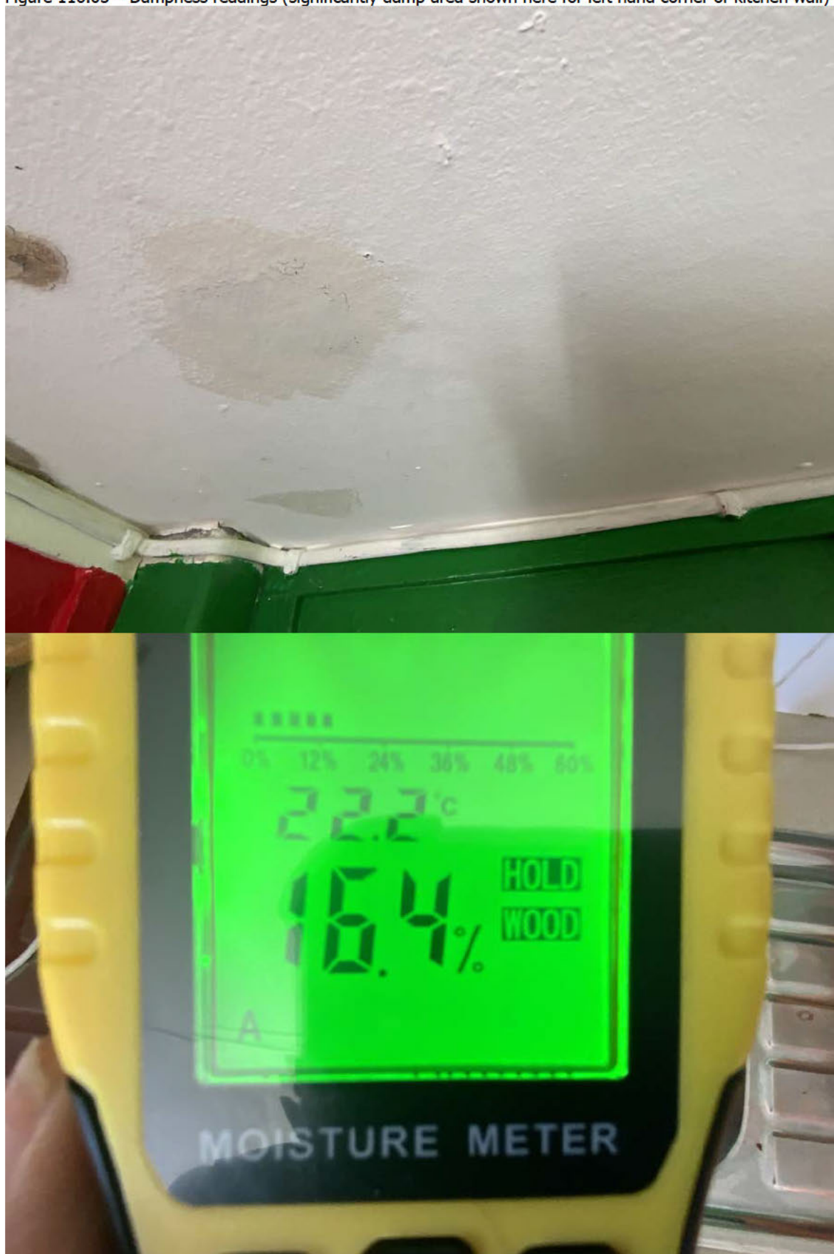
Figure 116.05 – Dampness readings (significantly damp area shown here for left hand corner of kitchen wall)
