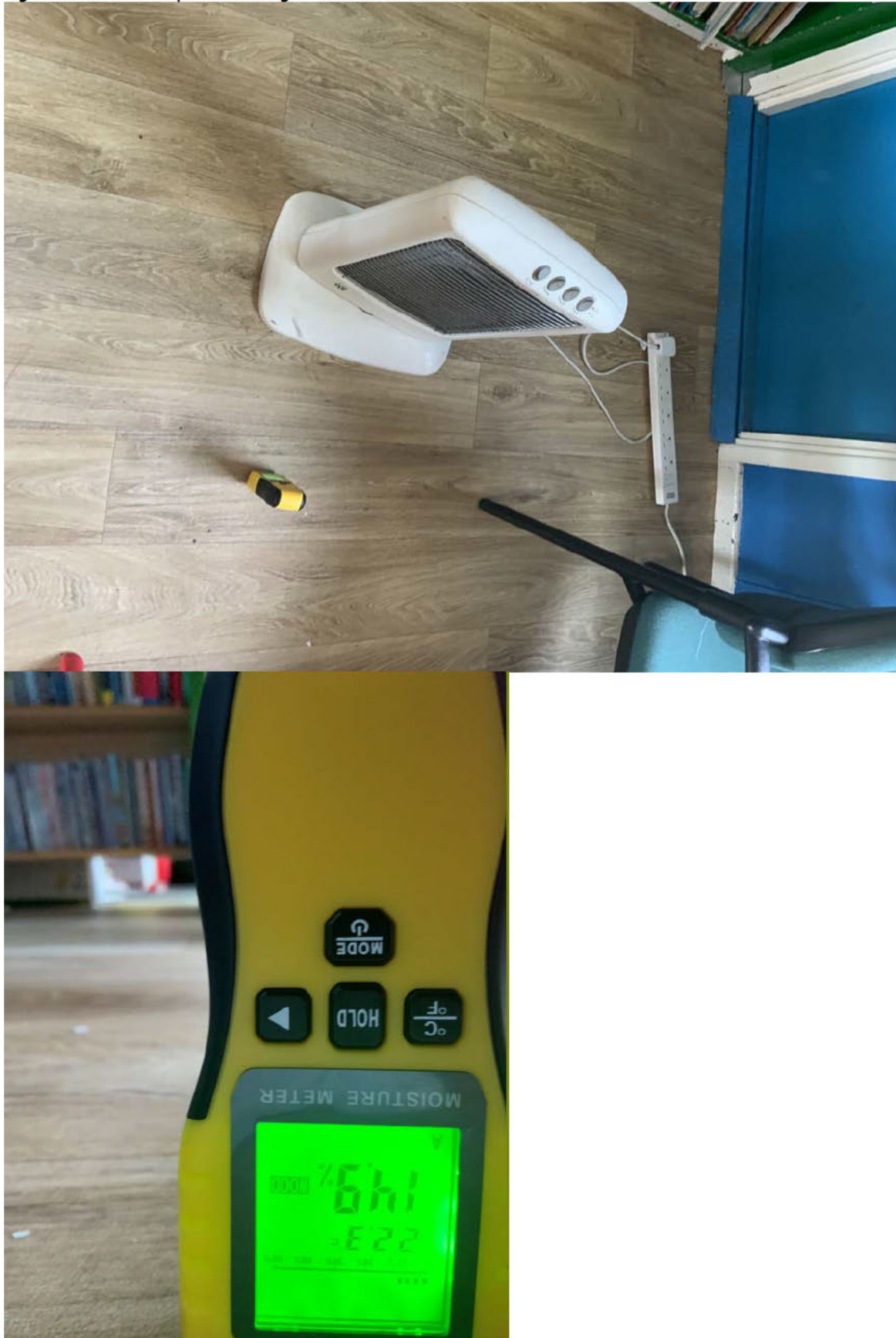
Figure 116.23 – Dampness readings – floor area with movement
