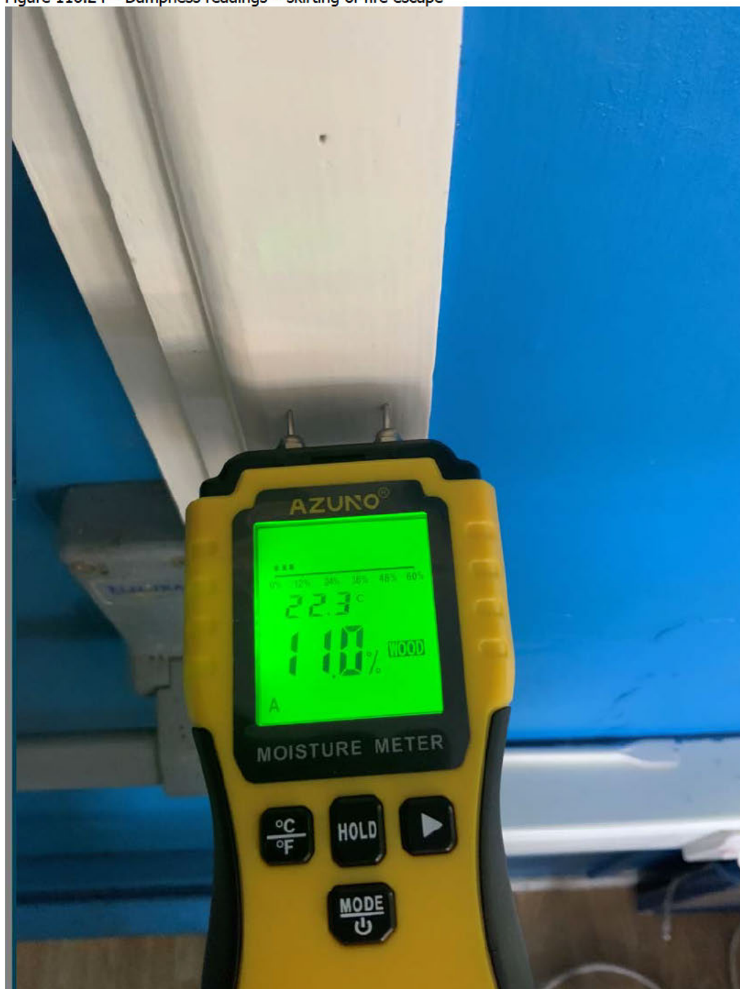
Figure 116.24 – Dampness readings – skirting of fire escape
