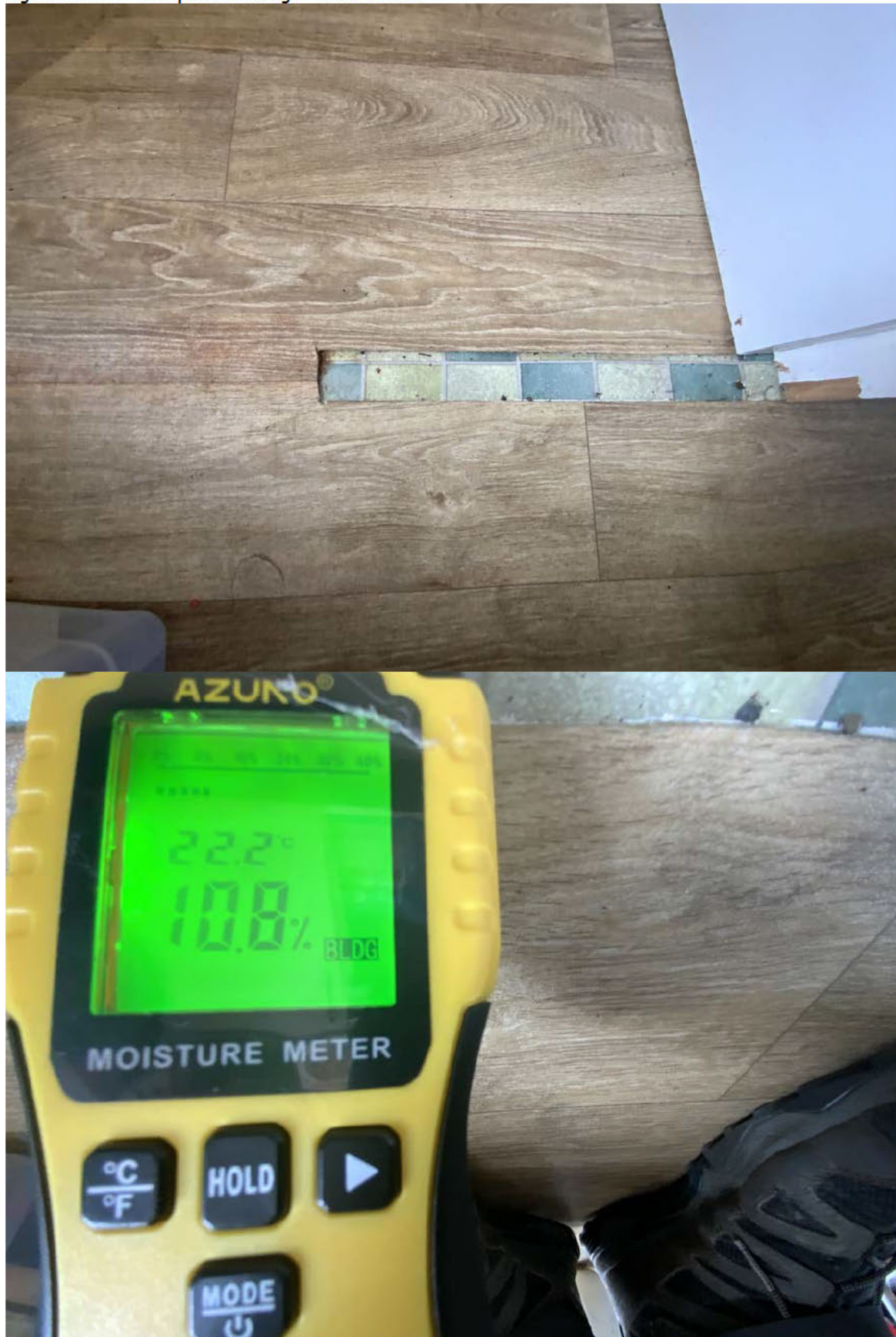
Figure 116.09 – Dampness readings – kitchen floor
