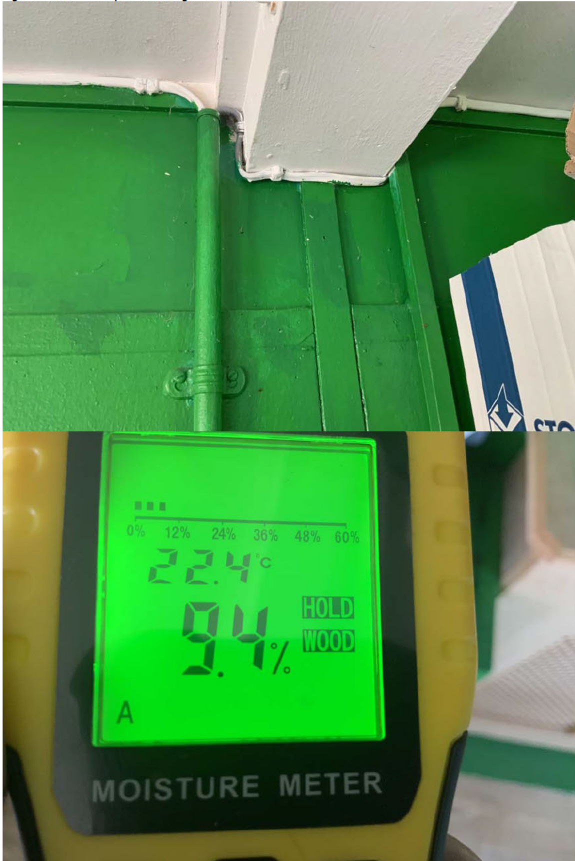
Figure 116.07 – Dampness readings – southwest wall
