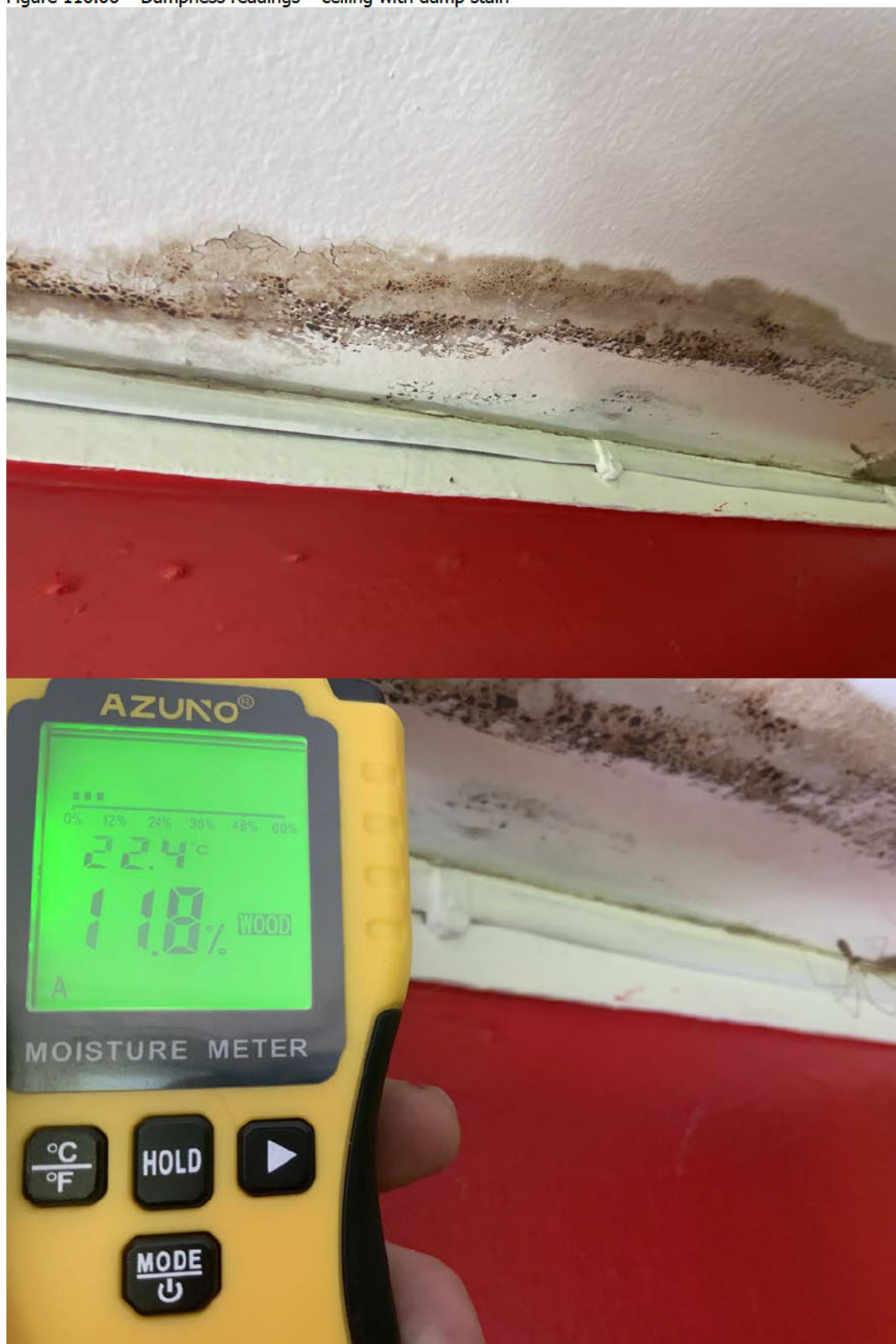
Figure 116.06 – Dampness readings – ceiling with damp stain
