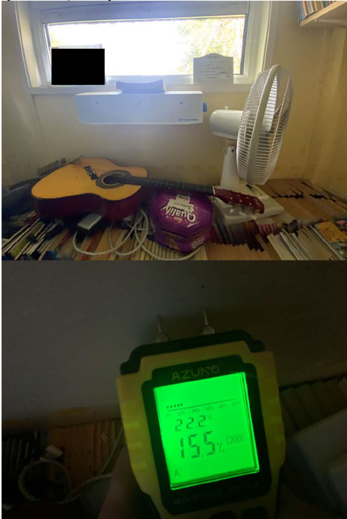
Figure 116.13 – Dampness readings – northwest wall toilet area
