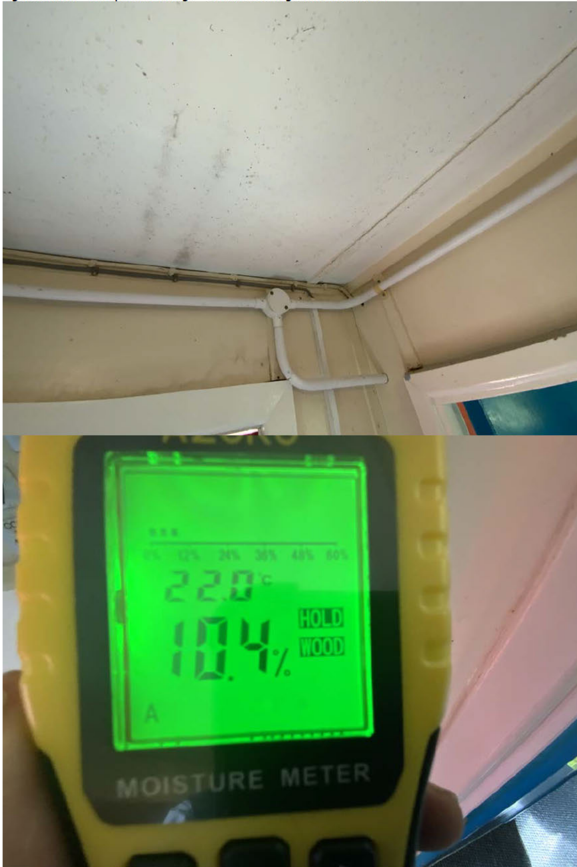
Figure 116.02 – Dampness readings – entrance ceiling black mould area
