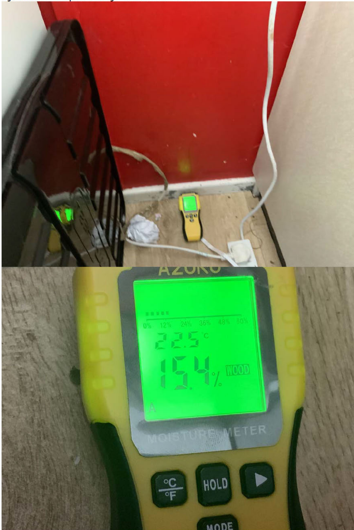
Figure 116.17 – Dampness readings – southwest wall kitchen area
