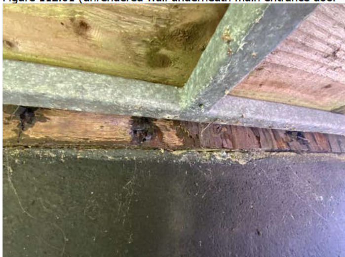
Figure 112.01 (unrendered wall underneath main entrance door – panel is rotten)
