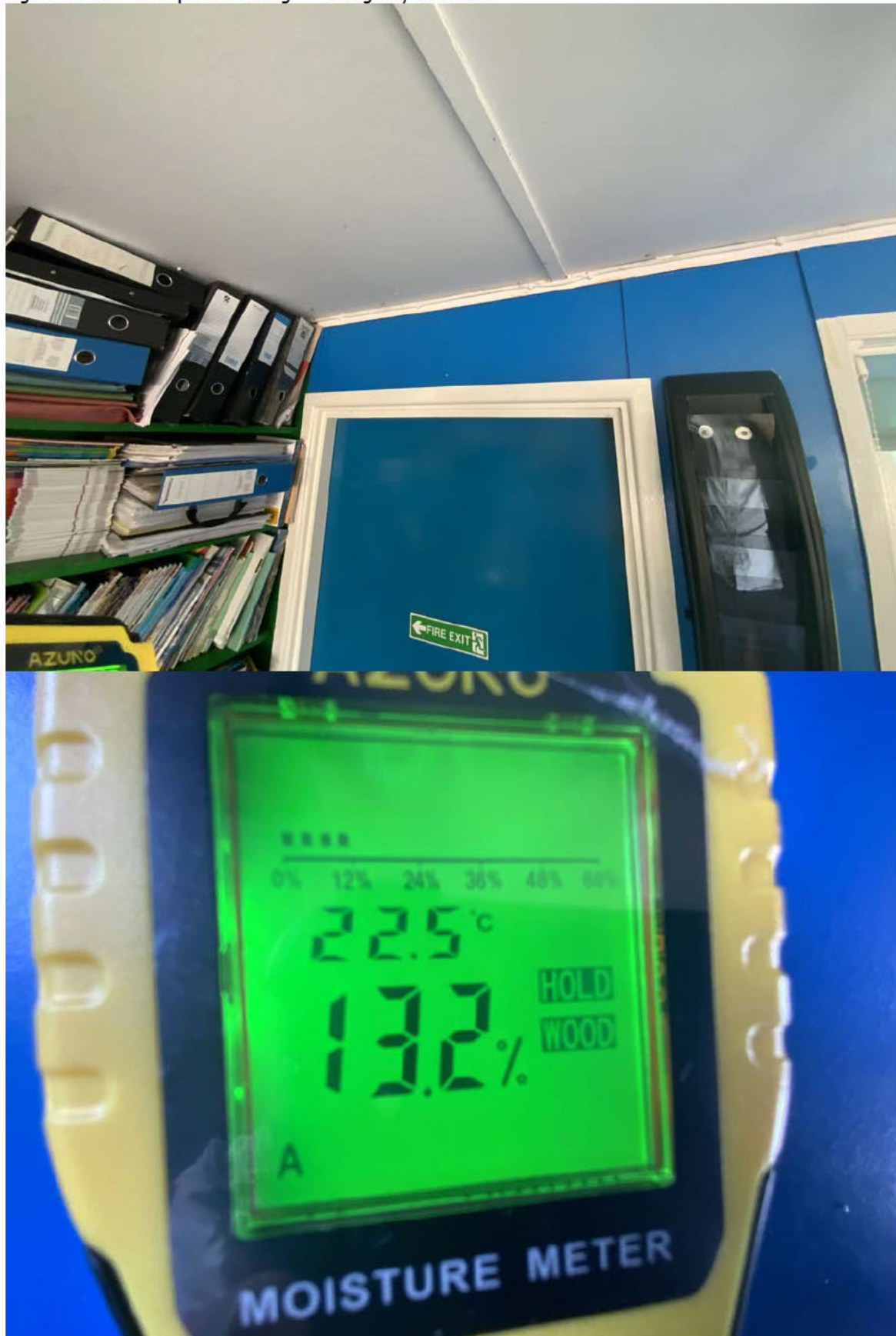
Figure 116.08 – Dampness readings – emergency exit wall
