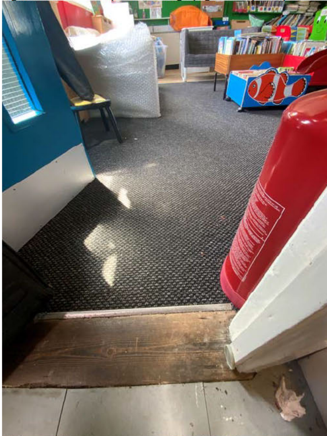
Figure 116.18 – Dampness readings (significantly damp area shown here in door saddles)
