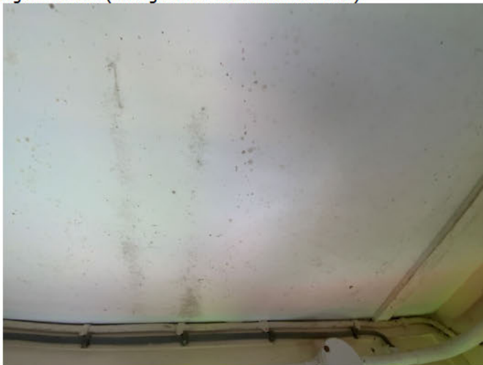
Figure 104.03 (ceiling at south corner of cabin – damp from roof outlet/internal downpipes)
