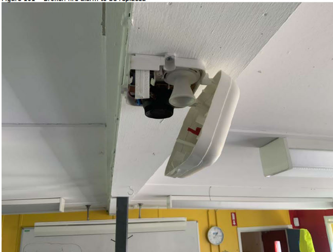
Figure 101 – Broken fire alarm to be replaced
