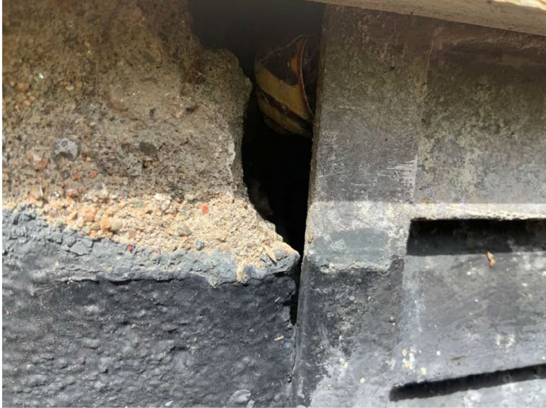
Figure 109 – Holes next to vent (southeast elevation next to gully) where pests may have access to floor
