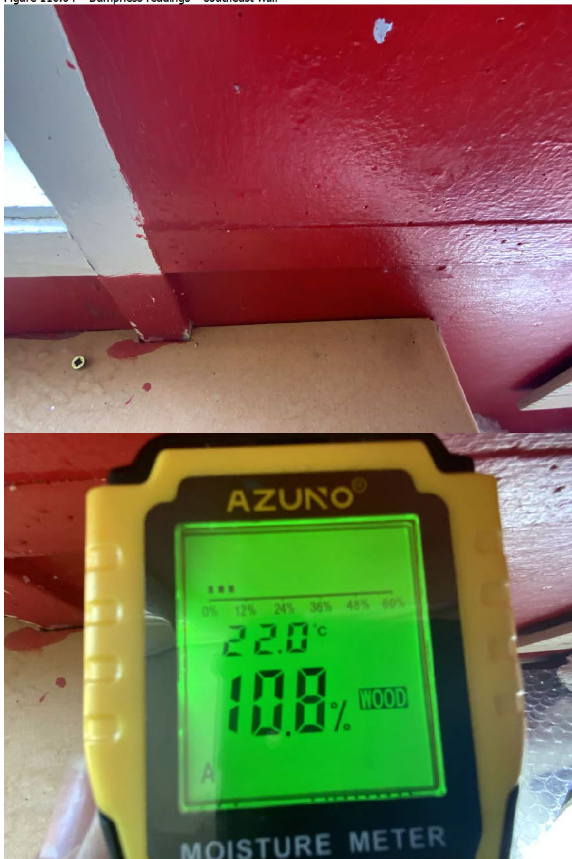
Figure 116.04 – Dampness readings – southeast wall
