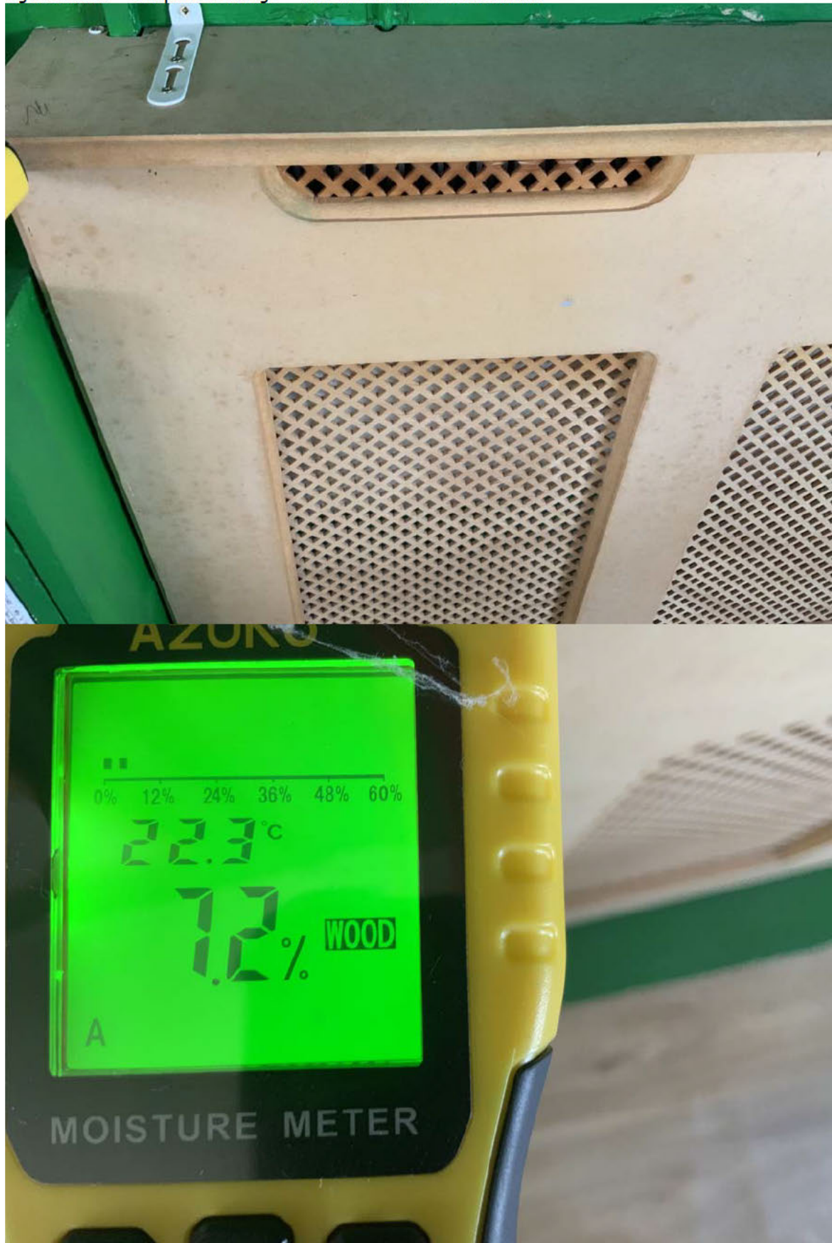
Figure 116.10 – Dampness readings – mdf enclosure of electric heater
