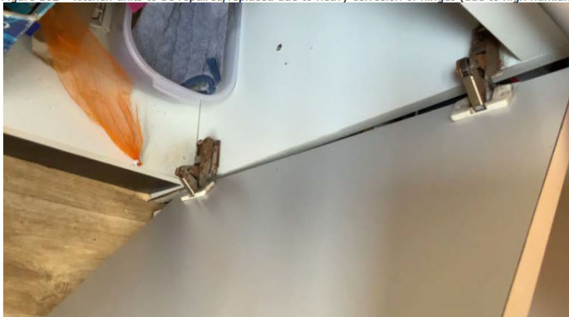
Figure 102 – kitchen units to be repaired/replaced due to heavy corrosion of hinges (due to high humidity)
