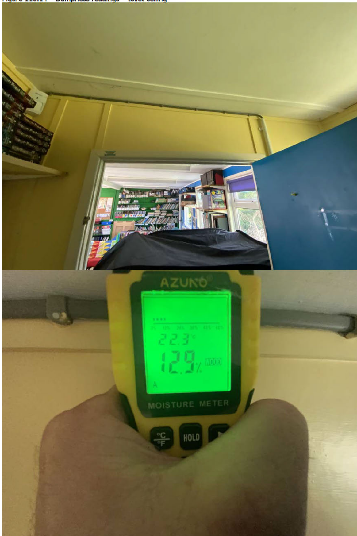
Figure 116.14 – Dampness readings – toilet ceiling
