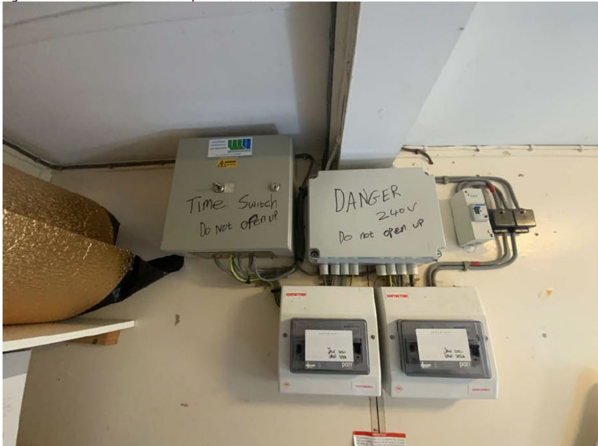
Figure 119 – wall mounted electricity switch boards
