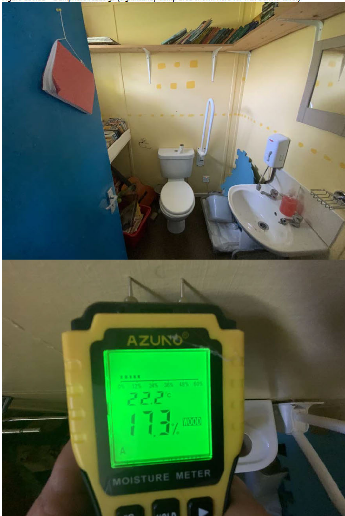
Figure 116.12 – Dampness readings (significantly damp area shown here for wall behind toilet)
