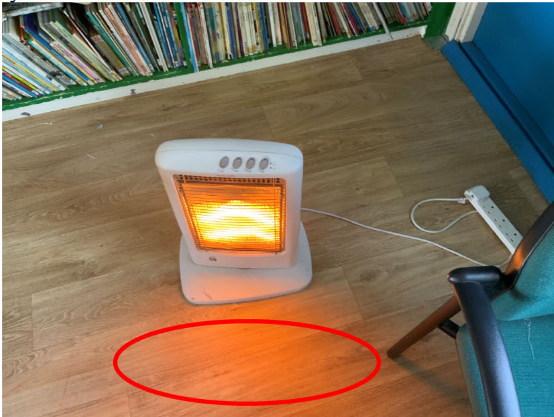
Figure 108 – Area of movement in floor in west corner
