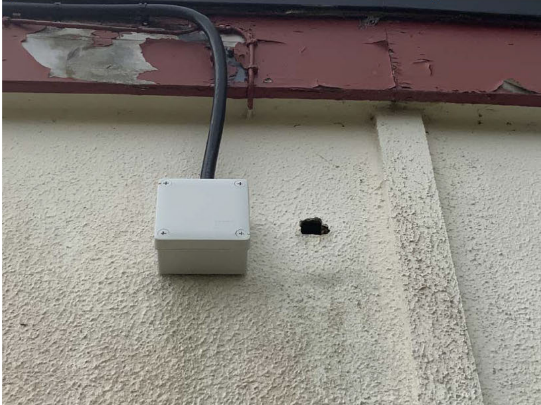
Figure 107 – Hole in wall on northeast elevation were birds have been seen nesting
