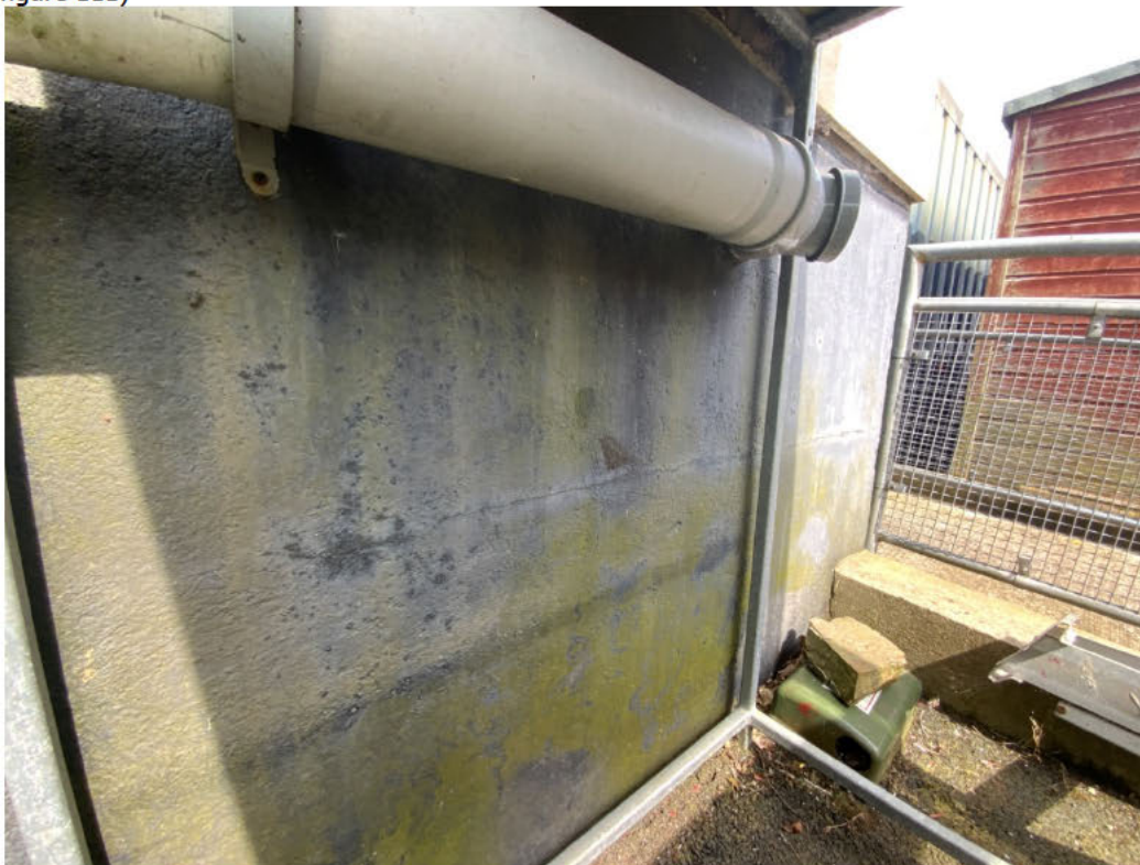
Figure 110.02 (southeast underneath stairs to main entrance – also shows broken pipe brackets as described in figure 111)
